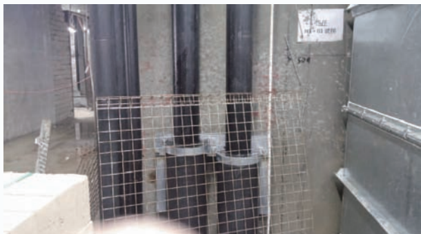
The pipe duct was fenced off to avoid falling from heights
